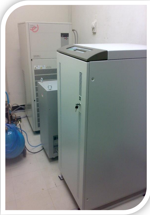
UPS 3:3 Phase 30KVA x1 Unit
